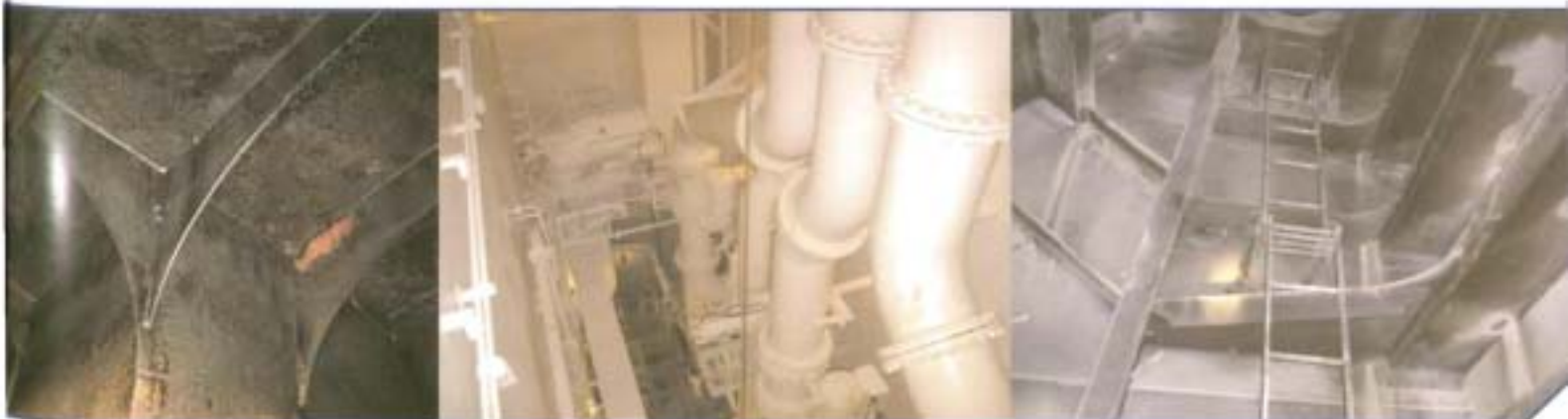
Inside Arosa 's cargo oil tank (left), engine room (centre), and water ballast tank (right) at 13 years of age.
